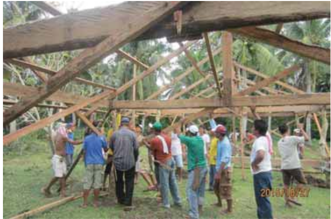
Building of structure where the Automated Coconut Sugar Cooking System will be installed in Ragay, Bicol, Camarines Sur
